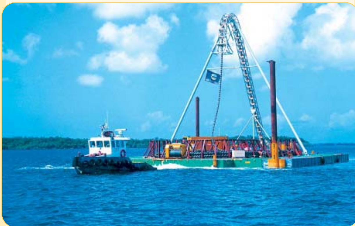
To enhance service reliability, Caribbean Utilities completed its first-ever submarine cable laying operation in 2001.
