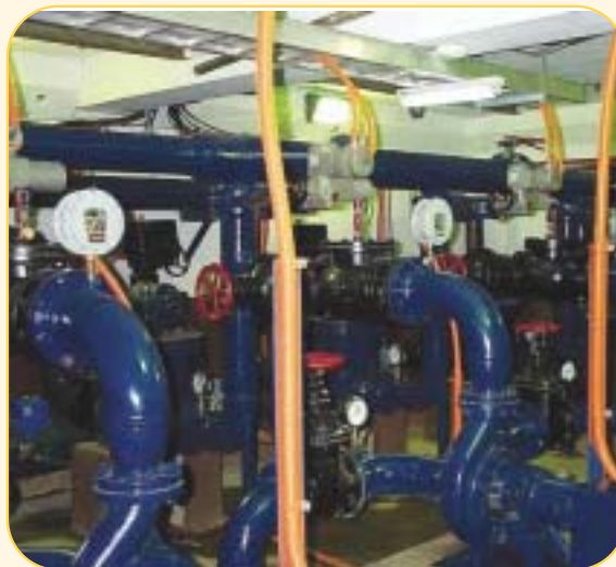
Equipment cooling water system
