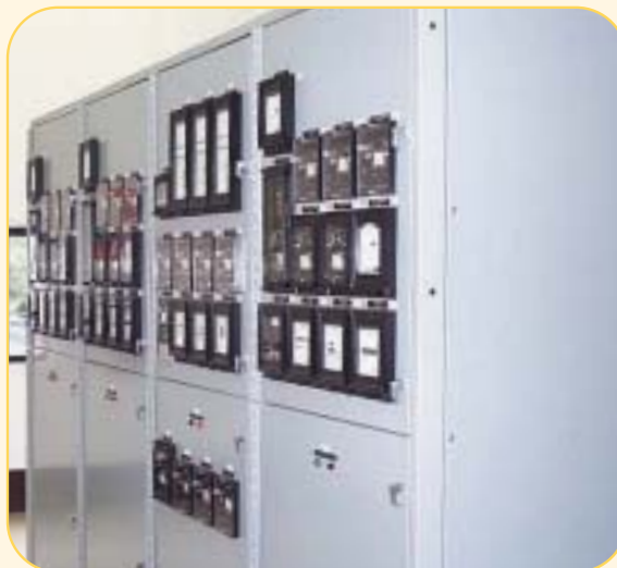
Control panel for Mollejon's three turbine generators
