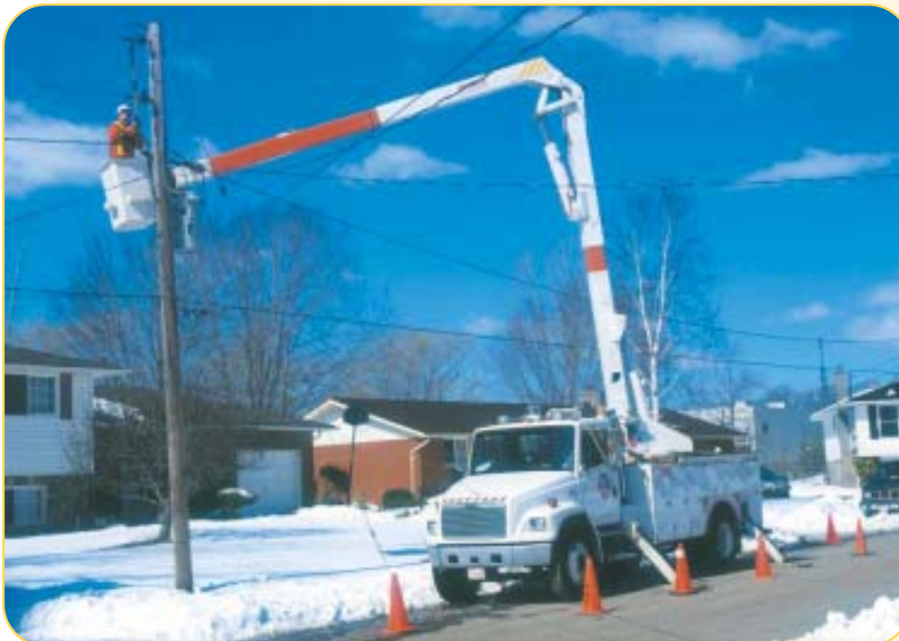
Canadian Niagara Power serves 15,000 customers in the Town of Fort Erie, Ontario.
